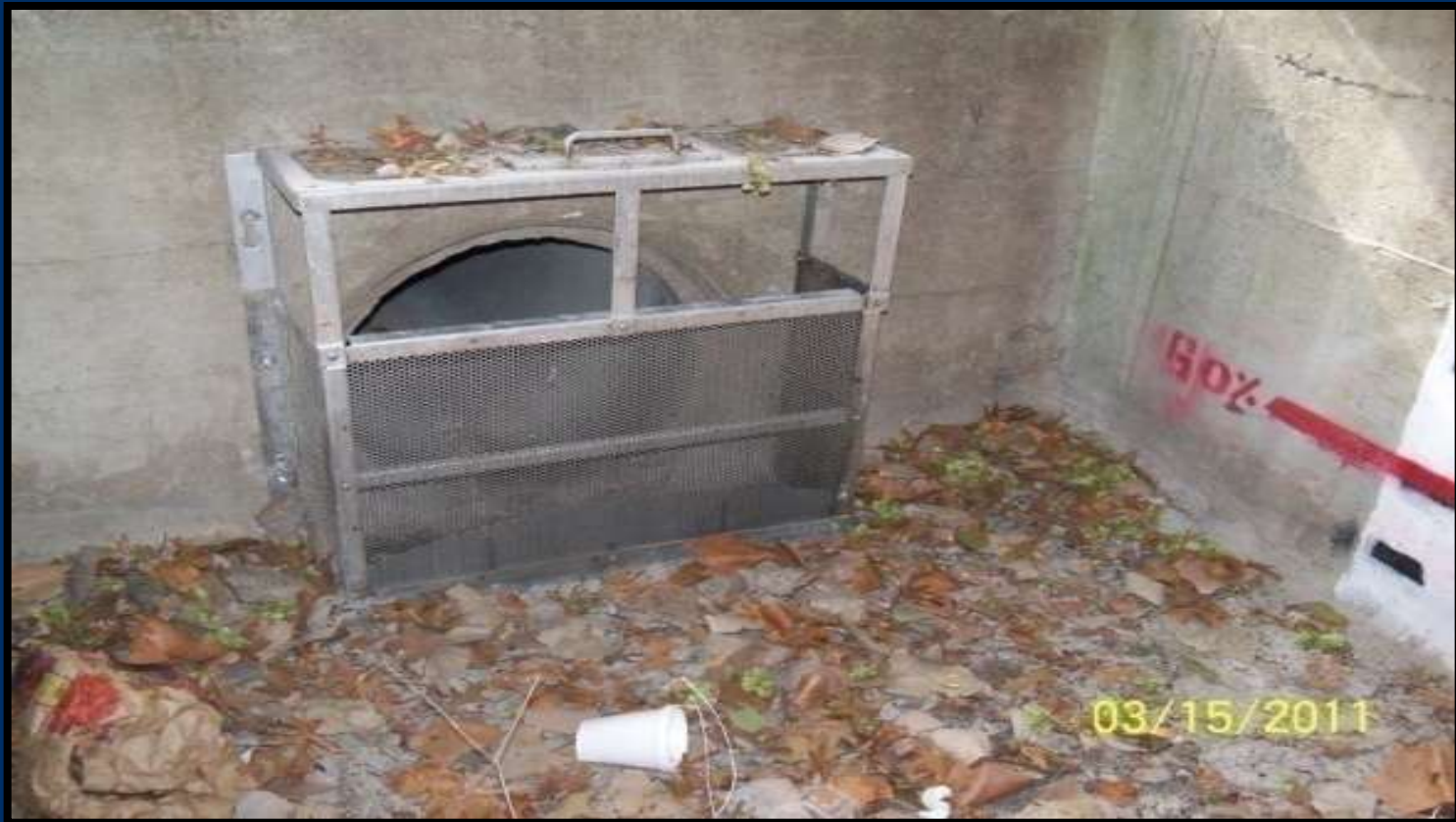
Connector Pipe Screen (CPS) inside catch basin/vault
